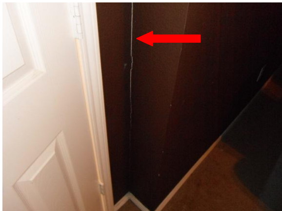
Vertical Cracks in Media Room
