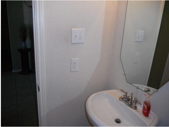
GFCI located in the hall bathroom
