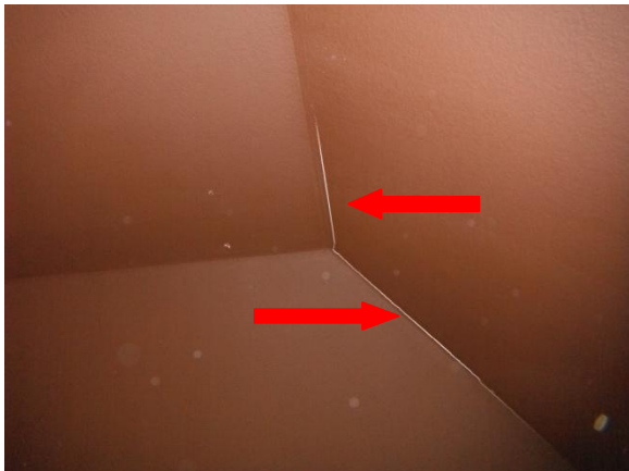
Crack in seam of drywall in Media Room ceiling
