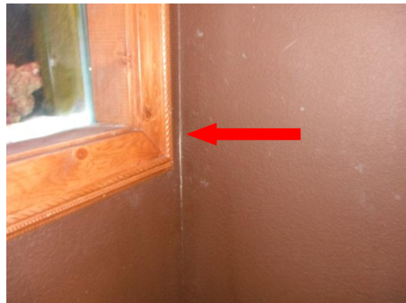
Vertical Cracks in Media Room
