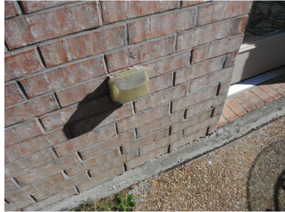
GFCI located in the rear of the house
