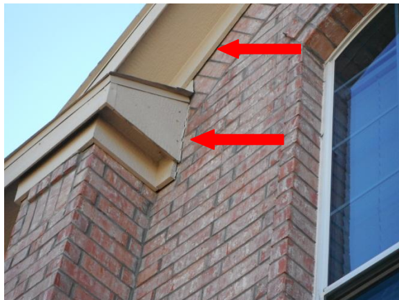
Evidence of cracks in the exterior trim
