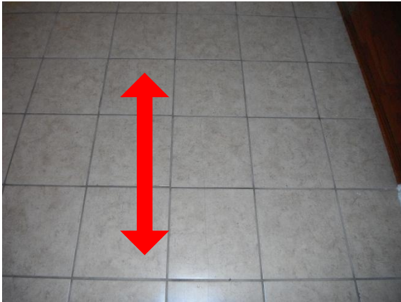
Foyer Tile shows continuous crack
