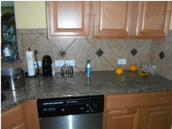
GFCI located in the kitchen
