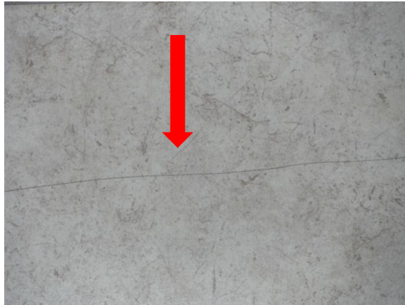
Foyer tile shows continuous crack
