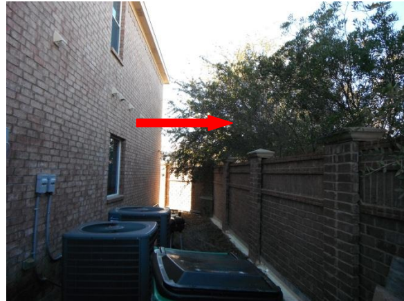
Overgrown Foliage on North side of house
