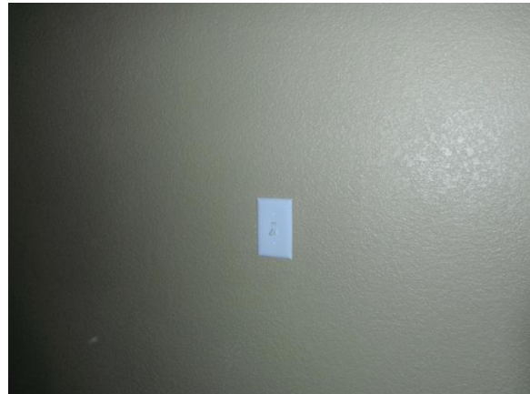
Wall switch located in the office not operating at the time of the inspection
