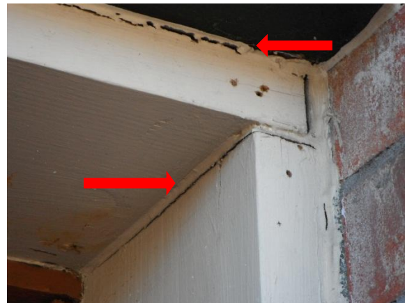
Evidence of cracks in the exterior trim
